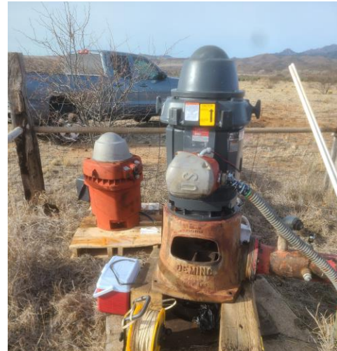
PHOTO 2 (2/23/25): New 50-hp motor and elevated pump column to aim discharge assembly north during testing (facing west).
