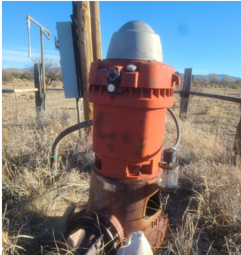
PHOTO 1 (2/19/24): Original motor found with significant damages to its wiring caused by a pack rat (facing east).
